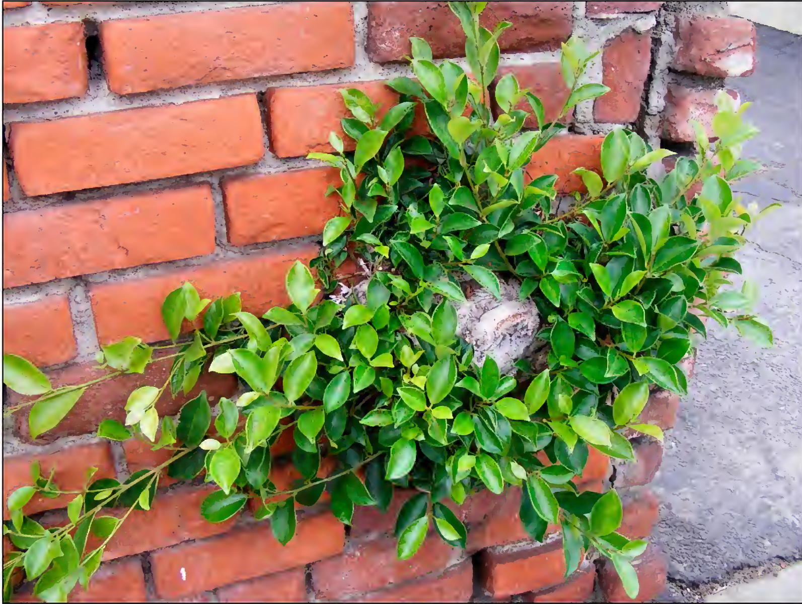
Figure 9. Ficus microcarpa grows in joints of old masonry and crumbling brick walls, Laguna Beach, Orange County. Note the base has been cut back during landscape maintenance activities.
